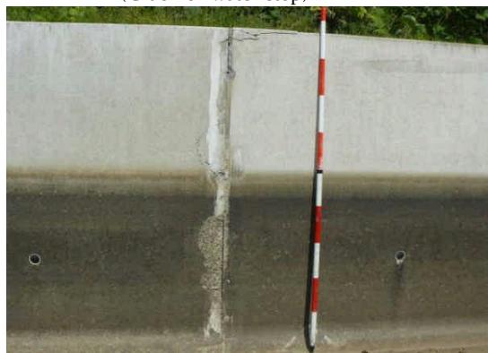
Fig.6 L型水路における目地部損傷 (Damage of joint part in L-type canal)
