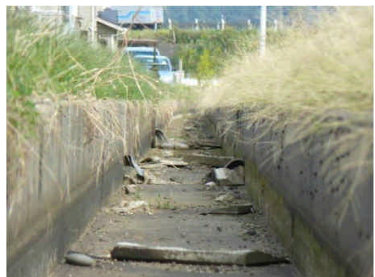
Fig.2 目地部が連続して損傷している状況 (Repeated breakage of concrete and collapse of water stops at successive canal joints)
