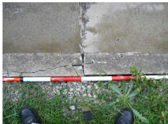
Fig.5 止水板の延長上に延びるひび割れ (Crack of water stop)
