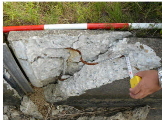
Fig.3 側壁が破損し鉄筋が変形・露出 (Concrete breakage and collapse exposing reinforcing at a canal joint)
