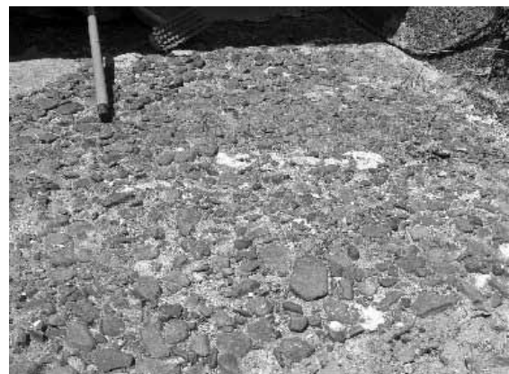
Fig.1 Abrasion at an irrigation canal
