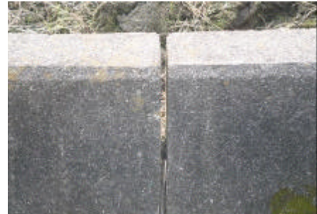
Fig.1 Defective Part of Canal Joiner
