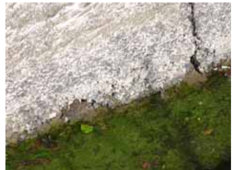
Fig.2 Corrosion and Leakage of Water
