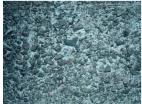
Fig.1 Abrasion by Water on Side Wall
