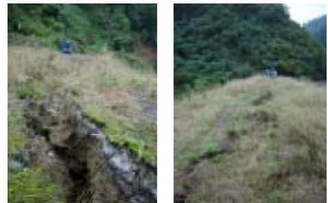
Fig.2 Damage of top surface
