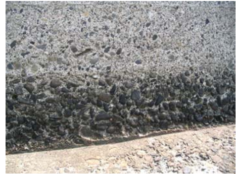
Fig.1 Abrasion of concrete canal
