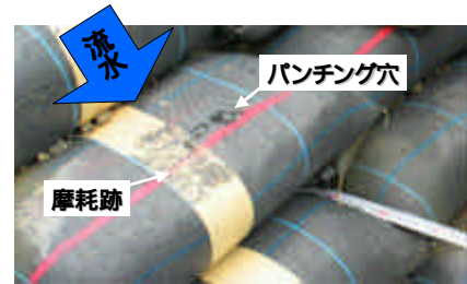
写真-1 土嚢材の摩耗とパンチング穴 Wear and punch holes on soil bag surface
