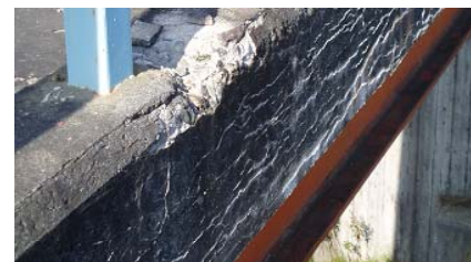
写真-2 附帯施設でみられた凍害ひびわれ Cracking of frost damage in attached facilities
