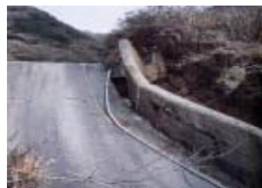
Photo 1 ため池洪水吐被災事例 Damaged Spillway of a Embankment
