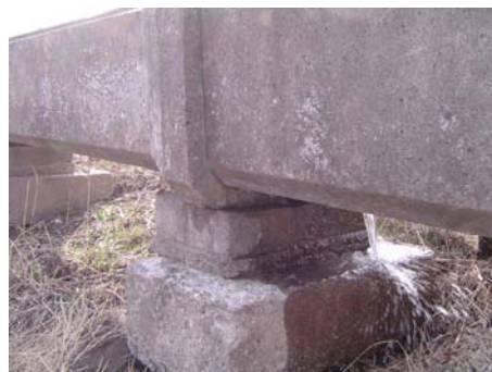
Fig.1 Water leak from joint of aqueduct
