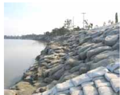
Fig.7 Sandbags on failed riverbank
