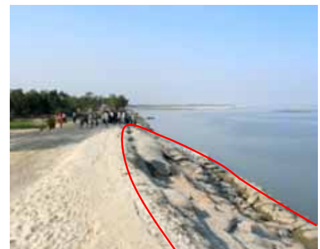
Fig.2 Failed Embankment of Jamuna
