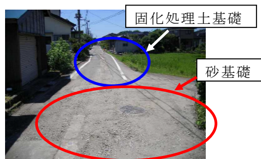
Fig.5 固化処理土で埋戻した区間と砂で埋戻した区間 An area backfilled by sand (front) and one backfilled by improved soil (back).
