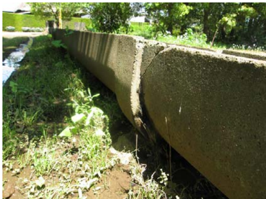
Fig.1 末端水路の目地部からの漏水 Water leak from joints for tertiary irrigation canals
