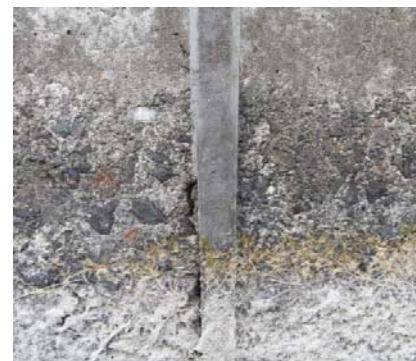
Photo 1 目地材の摩耗状況 State of erosion of joint sealant
