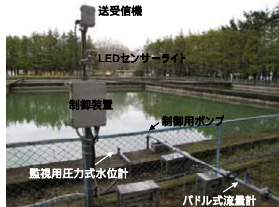
Fig.4 流量・水位・ポンプ運転監視制御用観測局 Observation point for supervisory control of water level, flow volume, and pumping operation
