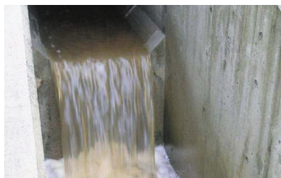
Photo. 1 An overview of the No.5 regulation pond and inflow loading through a box culvert
