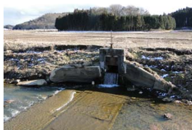
Photo 1 護岸の崩壊 Collapse of embankment
