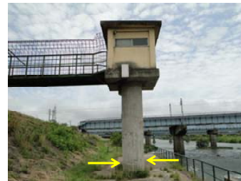
Photo 3 操作室の柱のひび割れ Crack at pillar of control room
