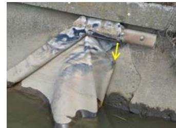
Photo 4 ゴム堰の袋体の端部亀裂 Broken end of rubber tube
