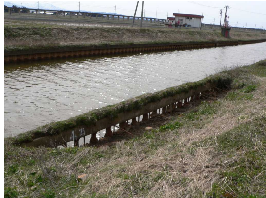
Pic-1 軽量鋼矢板護岸の腐食状況 Corrosion situation of light steel sheet pile
