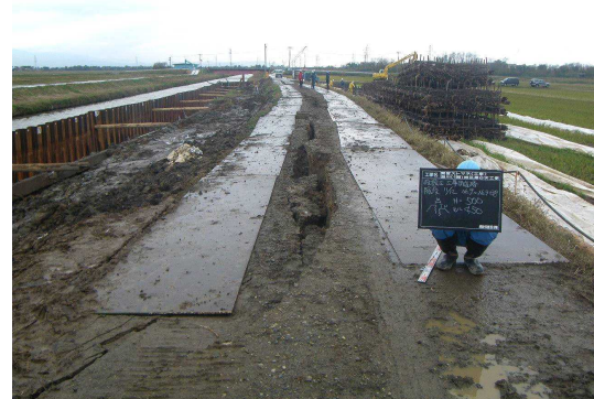
Pic-2 堤防すべり崩壊状況 Slope failure of the bank
