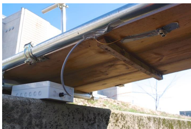
図3 観測装置の設置状況 Fig. 3 Placement of Observation Device
