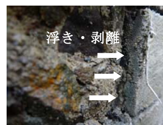
Fig.5 界面の浮き・剥離 Delamination of boundary
