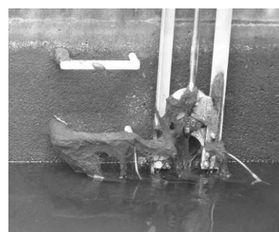
写真 2 分水工への藻類付着 Attachment of algae to division works
