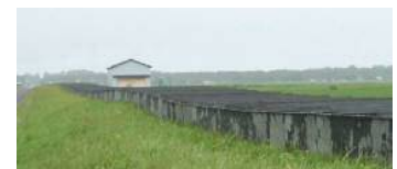
図 2 用水路の不同沈下状況 Situation of differential subsidence of canals
