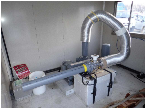
Fig.2 曝気ポンプの流量測定 Measurement of flow rate of aeration pump
