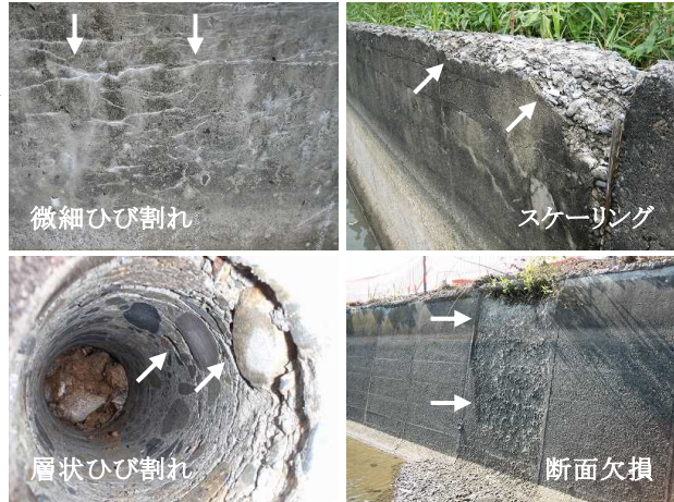
Fig.1 凍害劣化による代表的な変状 Typical deformation by frost damage deterioration
