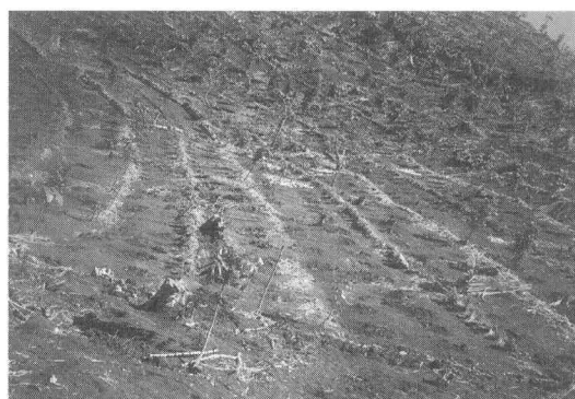
Fig. 5 Limestone walls together with Leucaena and Gliricida in Donomulyo village, Malang, Indonesia
