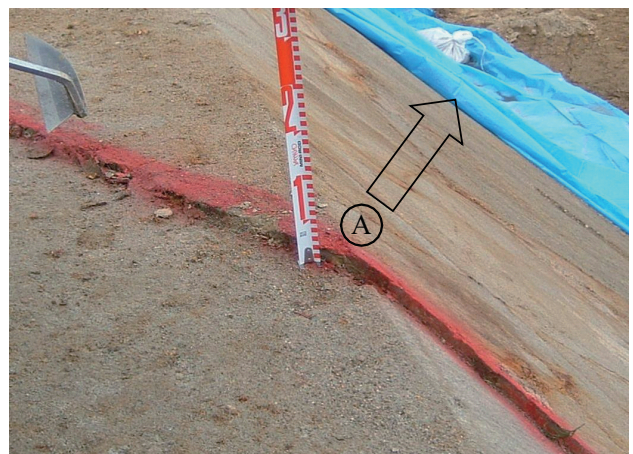
Photo. 1 膨張状況。 Situation of expansion.
