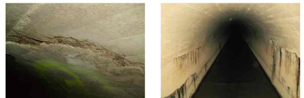
Fig.2 既設隧道状況 Decrepit tunnel
