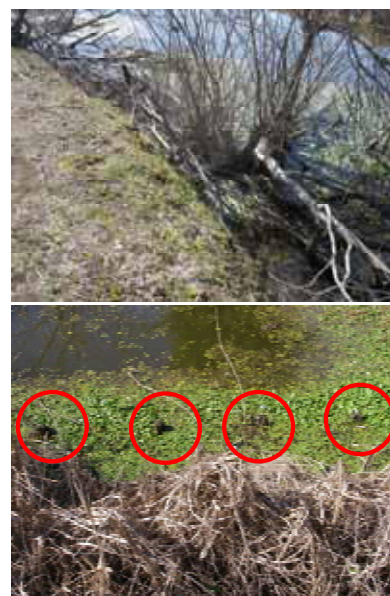
Photo.1 Degradation of soil-channel slope in Yanagawa city
