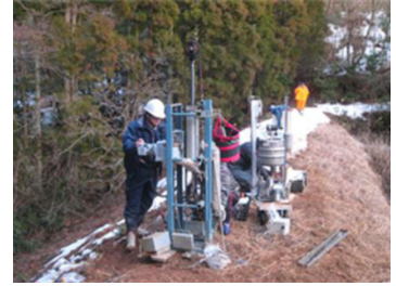
Fig.4 孔内回転せん断試験の状況 Photo of “Bore-hall Rotation Shear Test”
