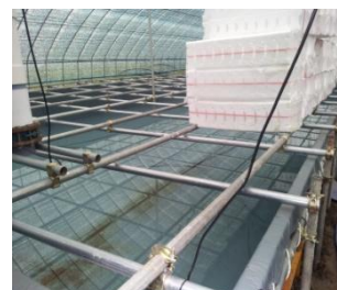
Fig 4. Rainwater tank, Gochang
