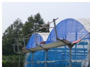
Fig 1. Rainwater canal in green house roof, Jeju
