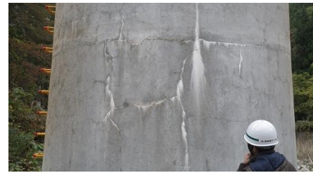
図1 吹付施工後の橋脚表面の亀裂 Fig.1 Cracks on the surface of the pier after repairing by spraying
