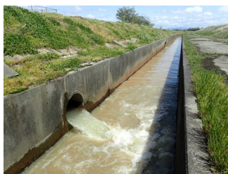
図-4 G揚水機場での余水放流の状況 Water delivery loss in G irrigation pumping station
