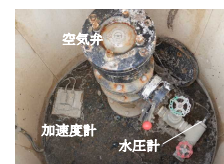
Fig. 3 計器の設置状況 Installation state of instruments
