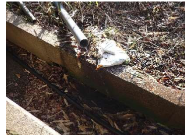
図5 漏水状況 (2022. 2. 10) Fig.5 Small amount of water leakage
